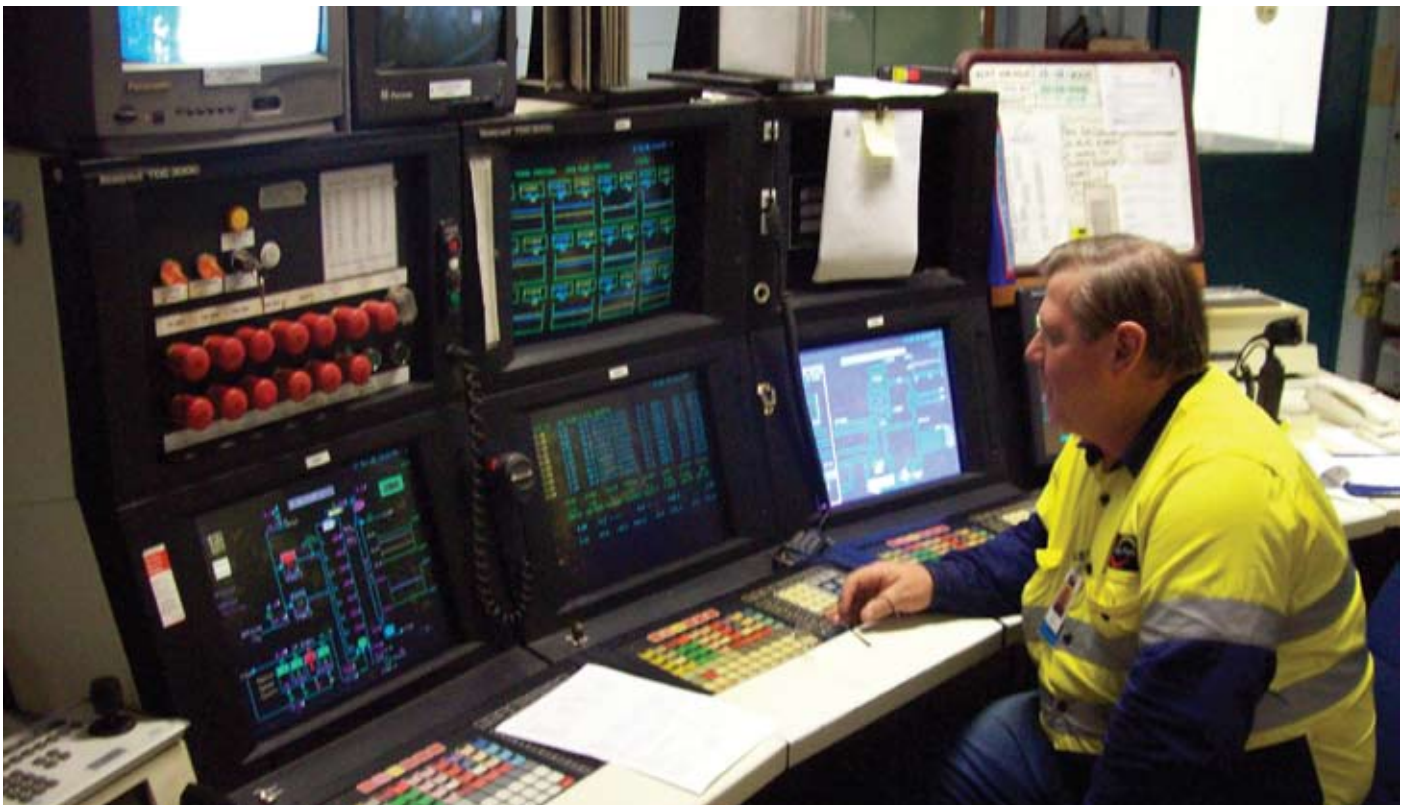
Control Room - Advanced Process Control
