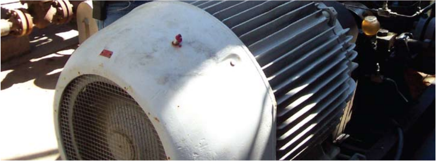
A motorised boiler feedwater pump
